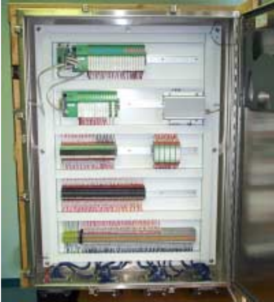
Figure 3 SCIU Assembly includes all I/O Points and power conditioning
